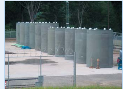
ISFSI Pad with new casks at IPEC. The smaller casks will be used for spent fuel from Unit 1 and the larger casks will hold fuel from Units 2 and 3.
